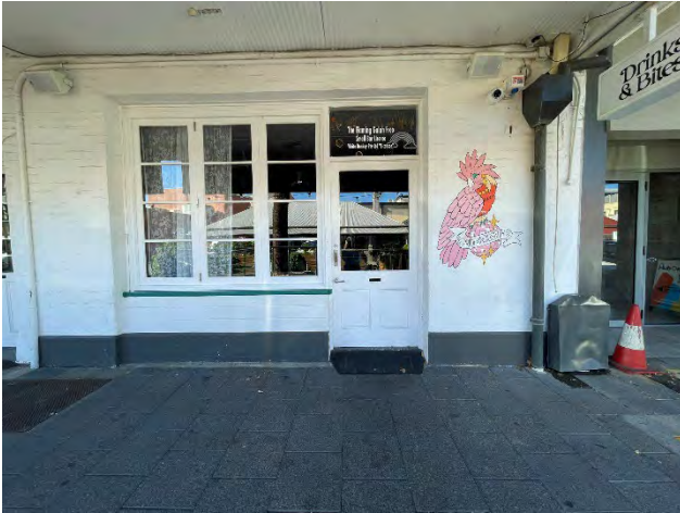
Figure 4: 19b Essex Street non original entrance.
