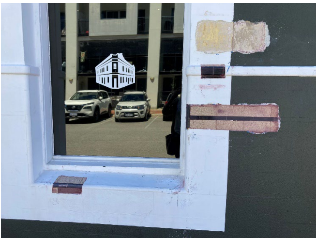
Figure 6: Materials investigation, Brisbane Street façade. Yellow square terrazzo dado tiles and black dado and sill tile edging ( dating from 1929) remain extant behind the top coat of paint. Source: Urbis 2025
