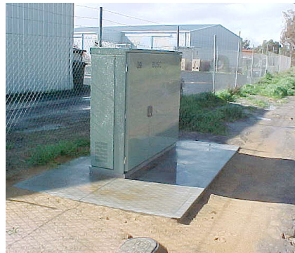
Remote Interface Module - industrial setting
