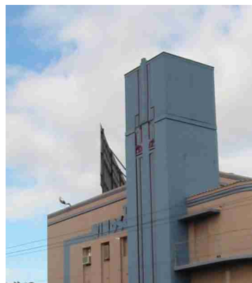
Antenna disguised as part of architectural feature (facade extension)
