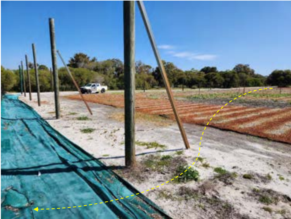
Plate 13: Western boundary of the site, at Lot 14, NE-SW direction. Previous drain filled and no surface water flow path through the site currently exists. Yellow arrow indicatively shows previous surface water pathway. Date of image: 09/10/2024
